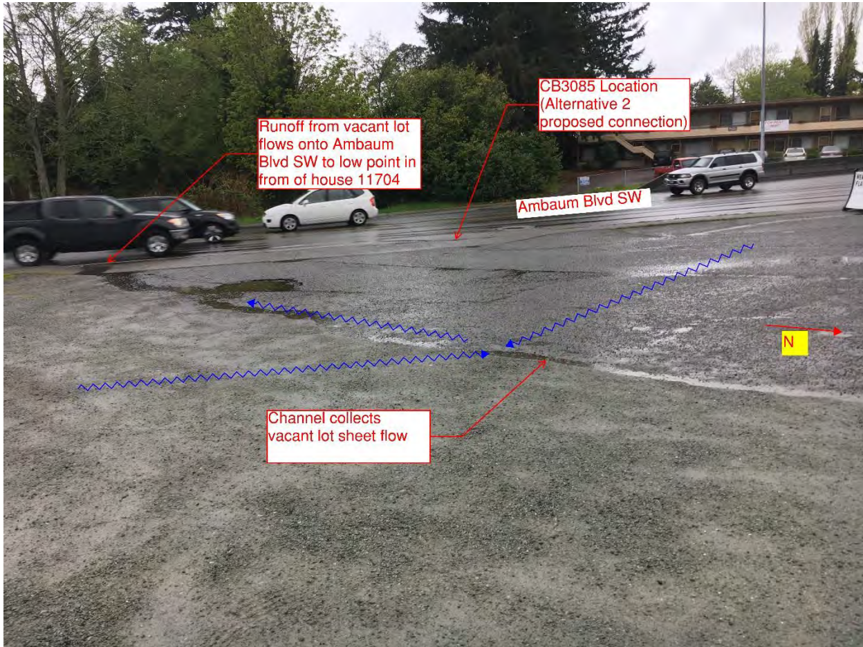
FIGURE 2: Sheetflow from vacant lot to Ambaum Boulevard SW north of issue location. Photo date 4/19/2019
