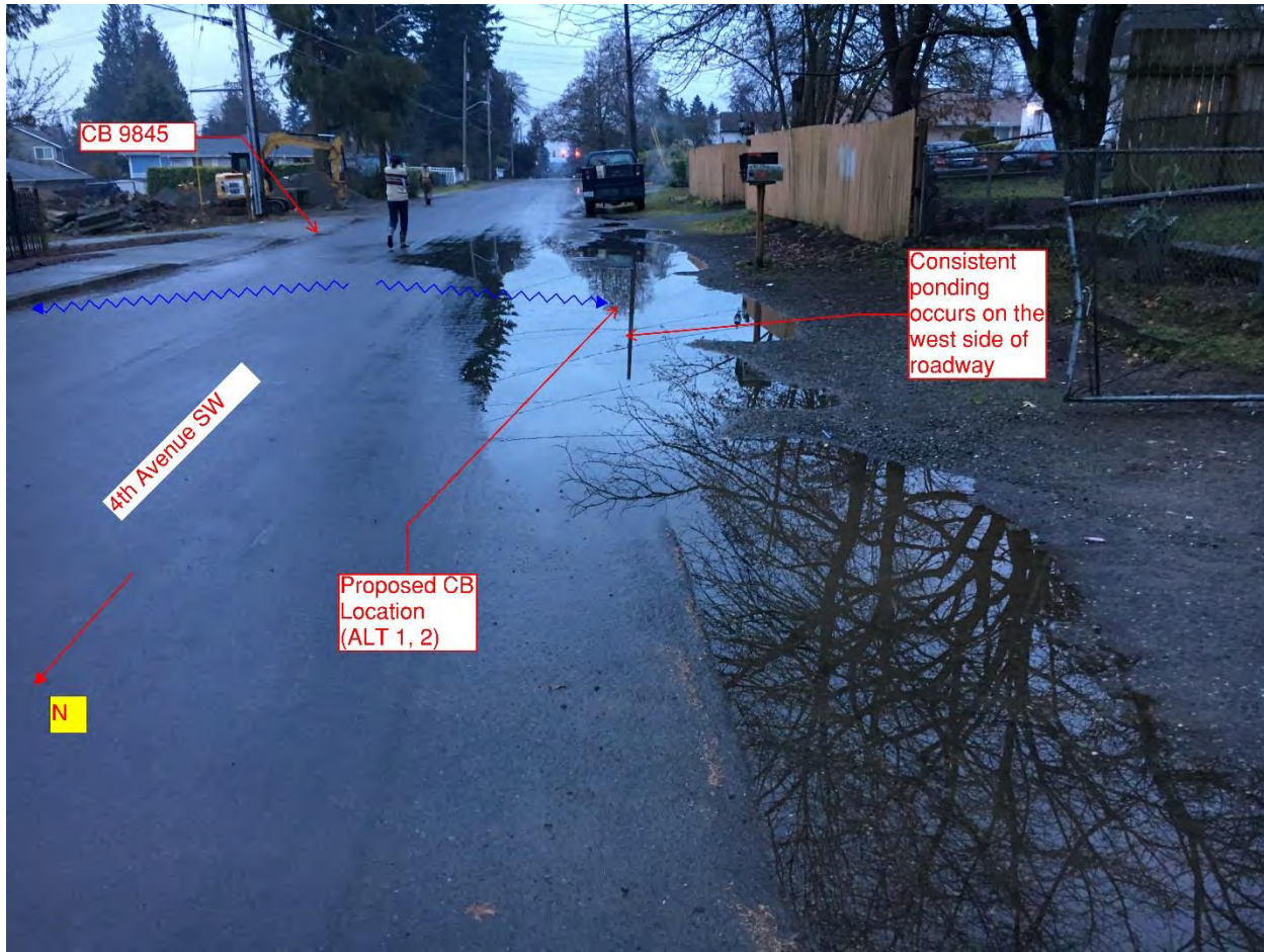
FIGURE 2: Ponding on 4th Avenue S, facing south. Photo date 3/12/2019
