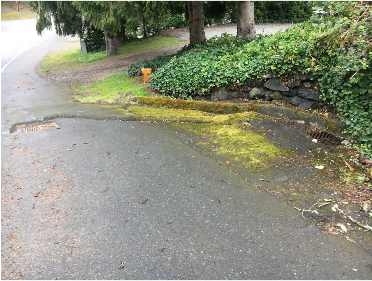
FIGURE 1: Looking northeast, picture taken 4/1/2019, CB2973 to the left and CB 7924 to the right, south side of SW 144 th Place, general flow direction towards northeast (flow from SW 144 th Place goes southeast into CB7924 which further drains northeast into CB2973).
