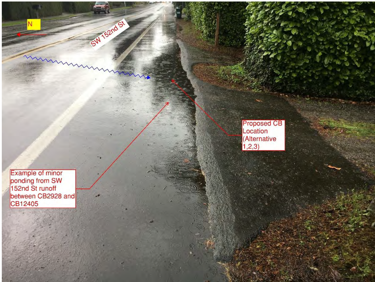
Figure 3: Small localized ponding in south shoulder of SW 152 nd Street. Photo date 4/8/2019
