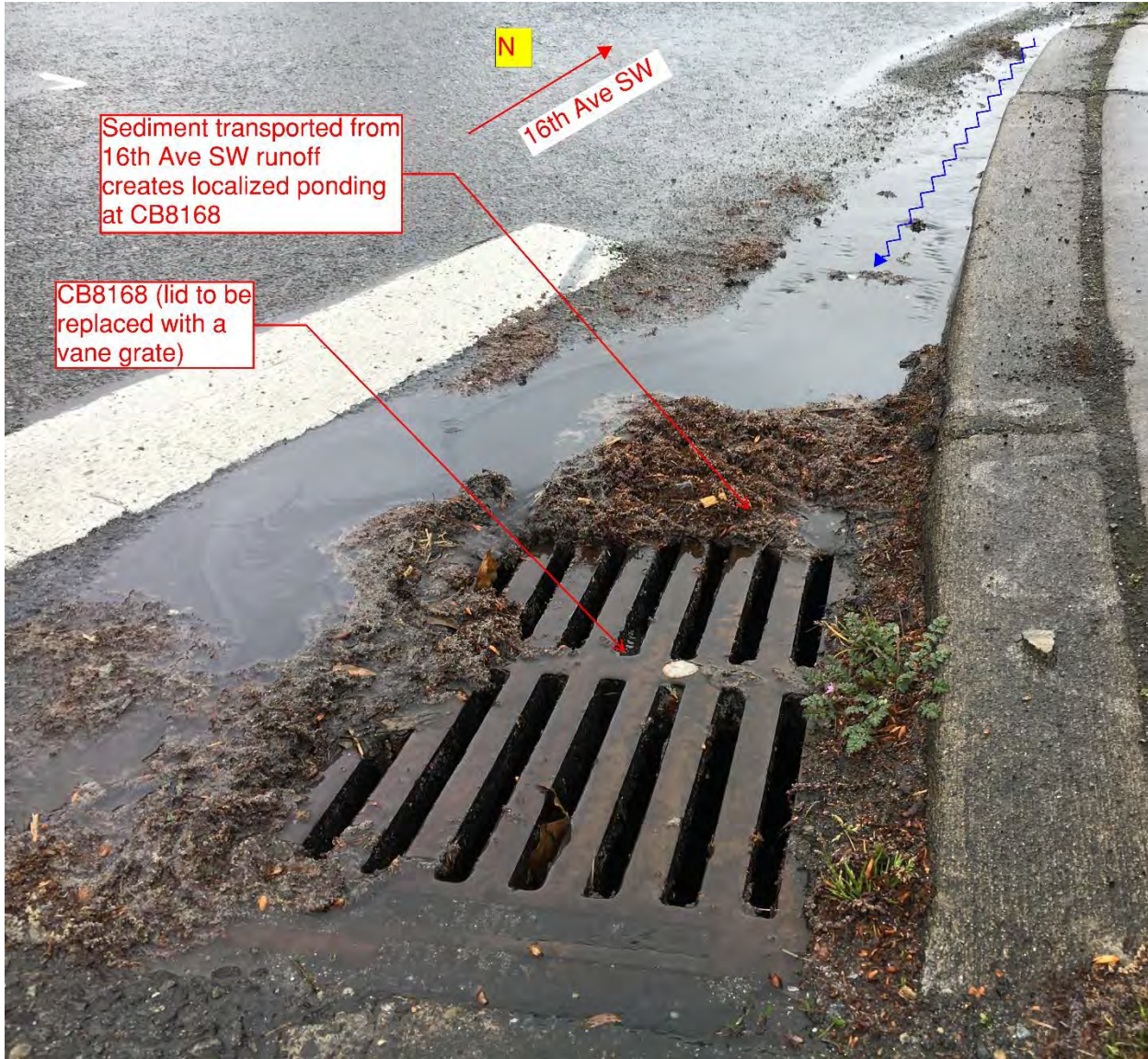
FIGURE 1: Localized ponding around CB8168 during small precipitation event. Photo date 4/8/2019, photo taken facing northeast
