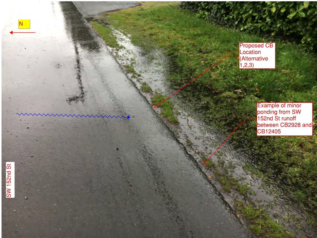
Figure 2: Small localized ponding in south shoulder of SW 152 nd Street. Photo date 4/8/2019
