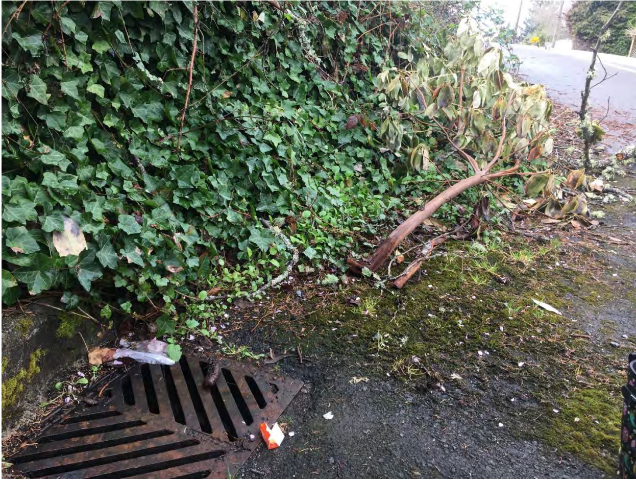
FIGURE 2: Looking northeast, picture taken 4/1/2019, CB 7924, south side of SW 144 th Place, flow direction towards southeast.
